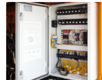
Centralized Electric Control Panel Large Electrical Cabinet allows easy access to the electrical components when maintenance or troubleshooting is required.
