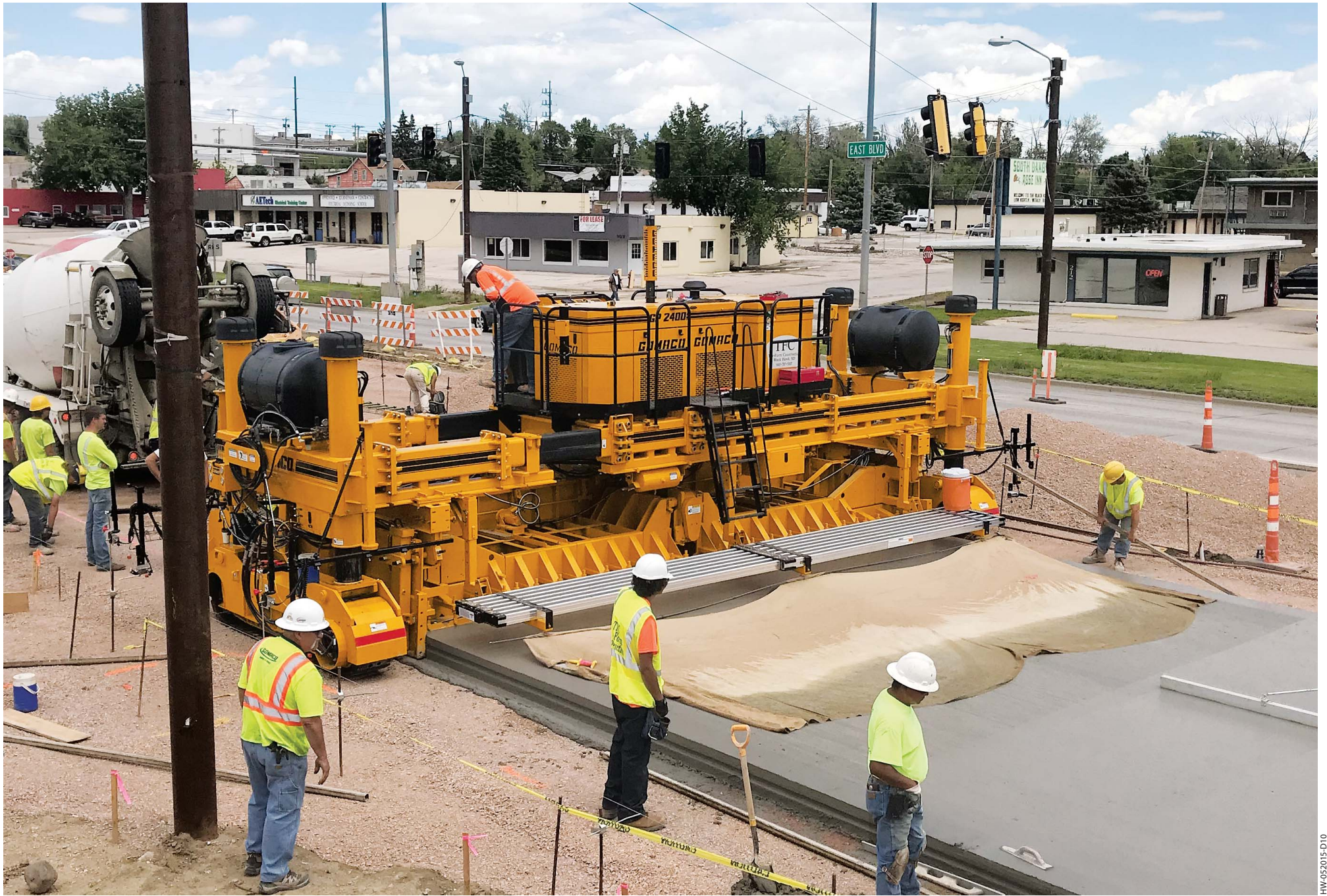
The GP-2400's ability to pave up to 24 feet (7.3 m) wide in tight, urban conditions makes it an ideal municipal paver. A two-track GP-2400 slipforms this new city street with a female keyway, in between existing obstacles.
