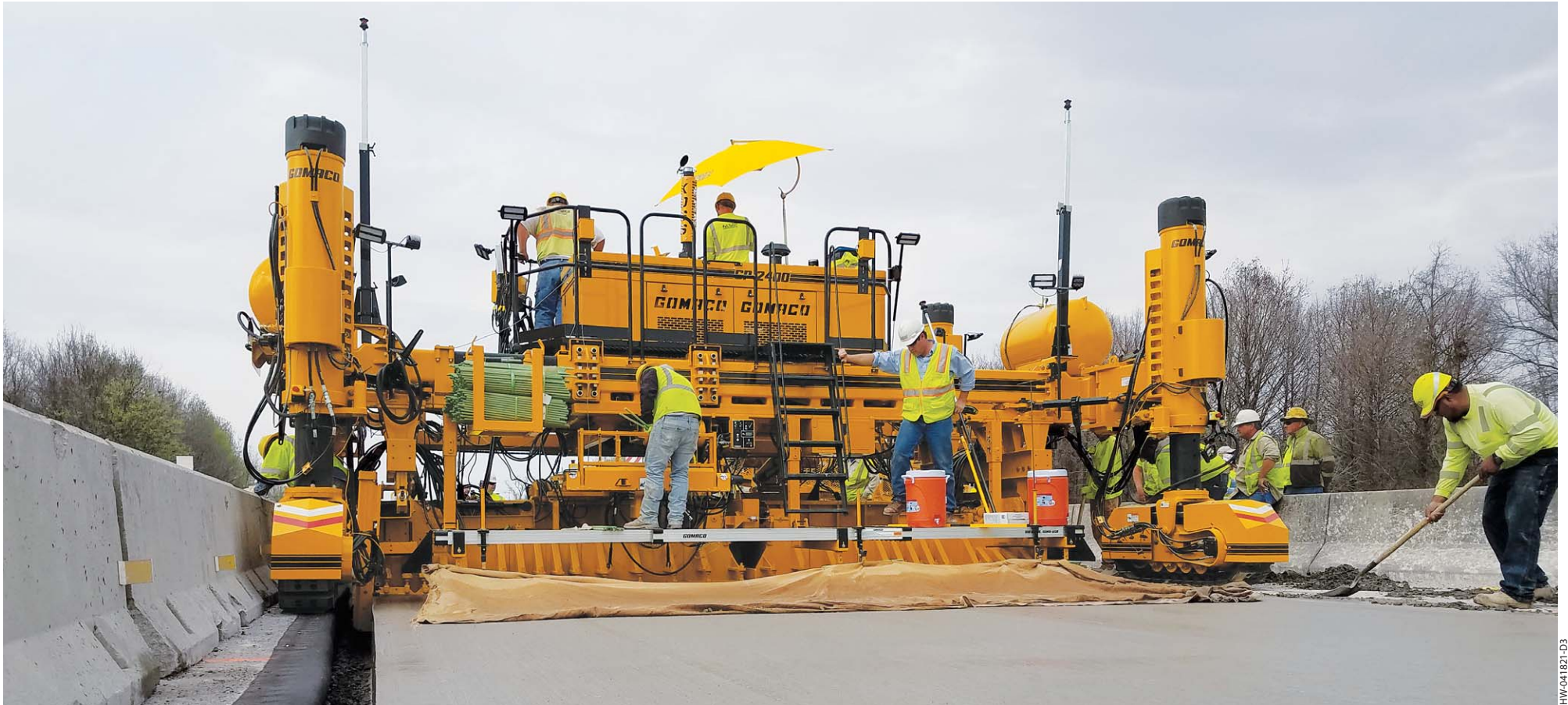
Minimum clearance is achieved with the four-track GP-2400 using 3D machine guidance to slipform a new interstate lane with existing traffic running next to the paving operation.
